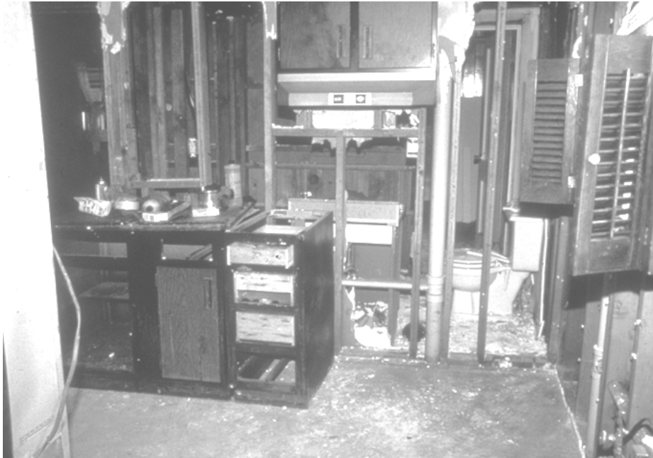
Figure 8-11. Even slow moving floodwater can cause substantial damage.
